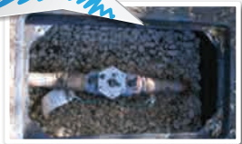
Double Check Valve Assembly on Irrigation System
