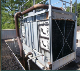
HVAC Units 15 Years of Service Life
