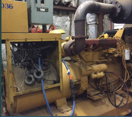
Generators 20 Years of Service Life
