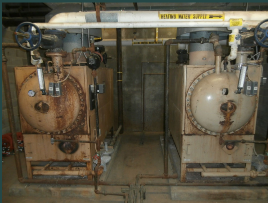
City Hall Boilers, original to building
