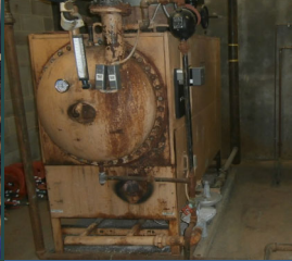
Boilers 25 Years of Service Life
