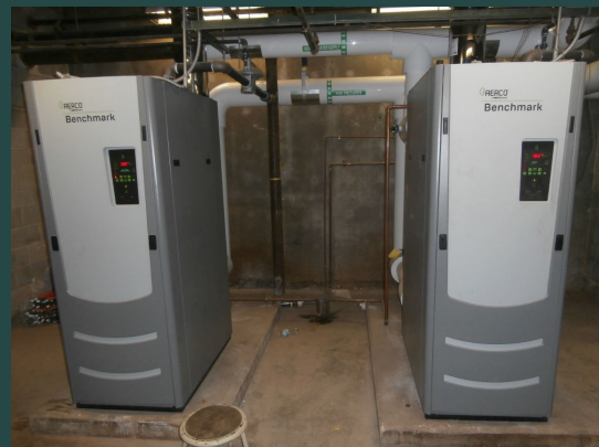
City Hall Boilers, new energy-efficient boilers Total Cost $311,000 in 2017
